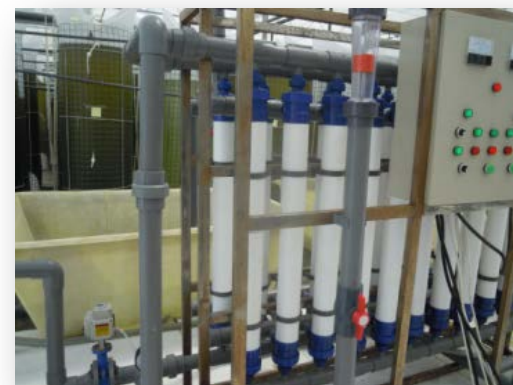
Picture of our installation with Flosep membranes
